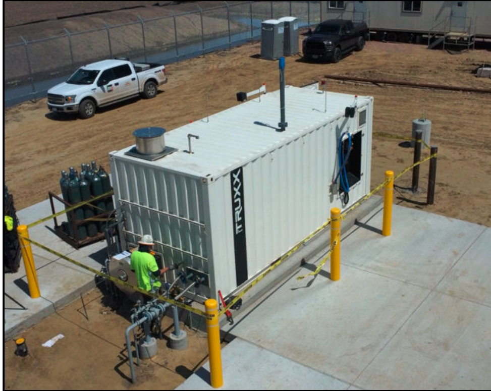
Existing RNG Decant Unit for Reference
